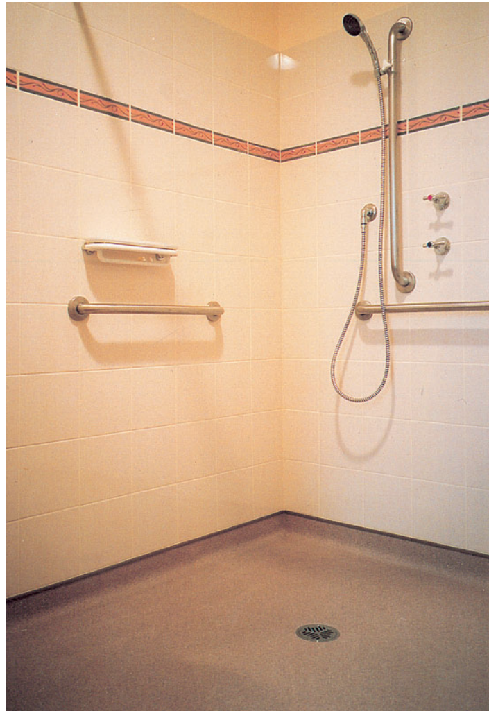
Cap Tile installed in conjunction with "Assurance" safety vinyl from Spectrum Floors
